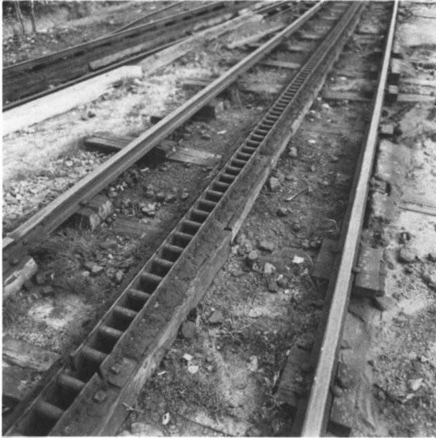
Figure 25. Closeup of the Cog Railway's running rails and the central cog rail which receives the cog gear positioned underneath the locomotive, 1994. Photo by the author.
