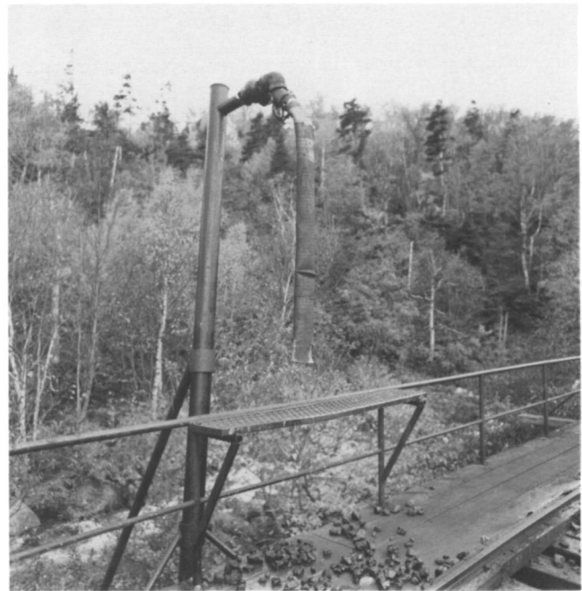
Figure 27. The hose at the Base Station used to fill the boilers with water, 1994. Photo by the author.
