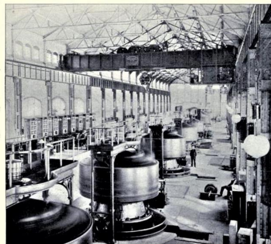
50-TON TRAVELLING CRANE. IN POWER HOUSE OF NIAGARA FALLS POWER CO.
