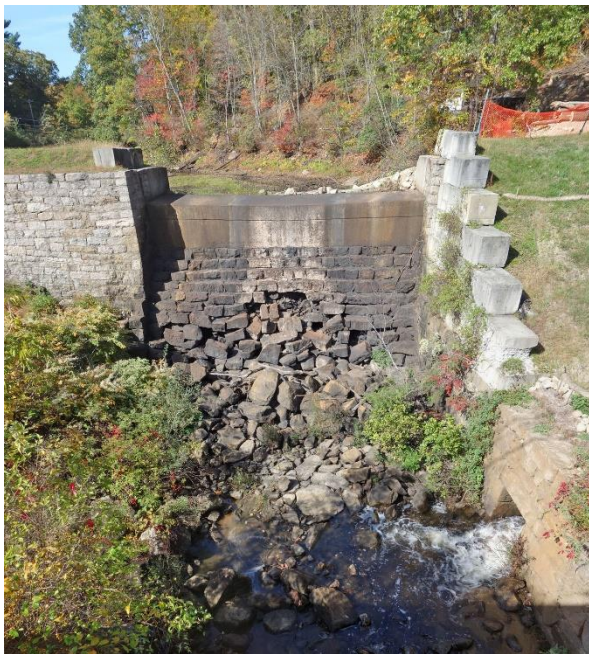
2020 view northwest of principal spillway, and low-level drawdown outlet (lower right). (Michael Raber)
