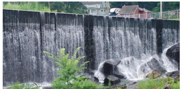
Leaking dam c 2020. (No attribution)
