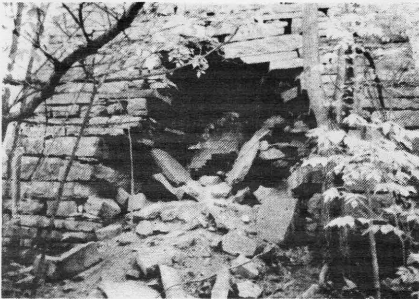
Figure 2. A 1986 photo showing the damage to the casting arch 30+ years after the wall was dynamited (Rolando photo).
